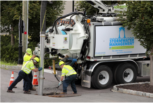
Above: WWSA crew vacuums water and debris from stormwater catch basin in Edwardsville.
