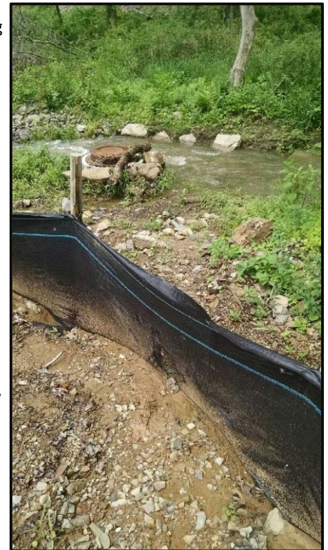
Figure 8: A damaged silt fence which is supposed to provide erosion and sediment control where soil is being disturbed by construction (Source: Allegheny County Conservation District)
